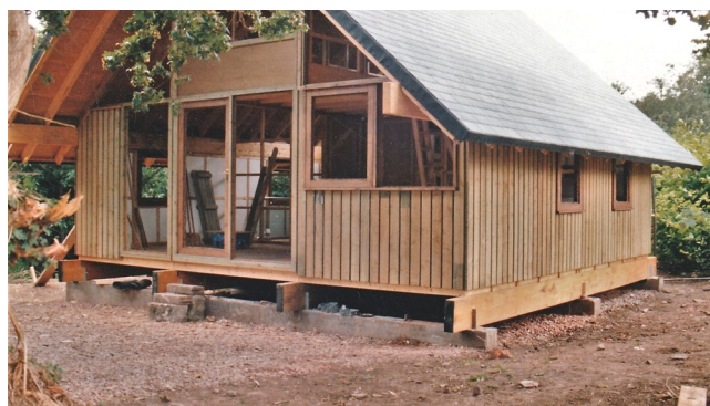
The kit building under construction in 1988 - it was one of several designs drawn up as holiday homes for the Forestry Commission.
